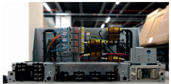
Rear view of withdrawable unit
